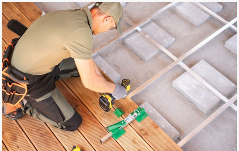
A worker focused on deck installation using power tools to secure patio flooring on a wooden deck.
