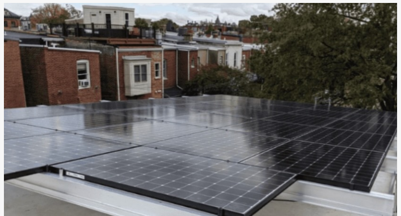
District Energy LLC Rooftop Solar
