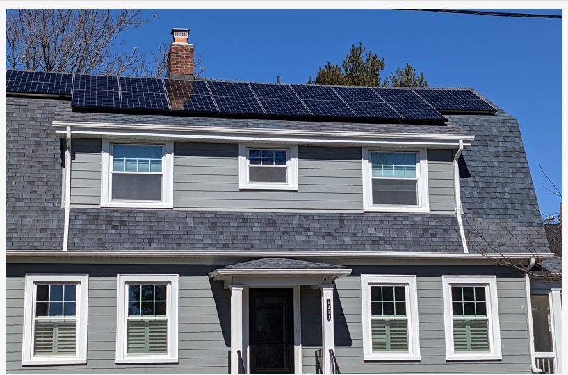
District Energy Residential Installation
