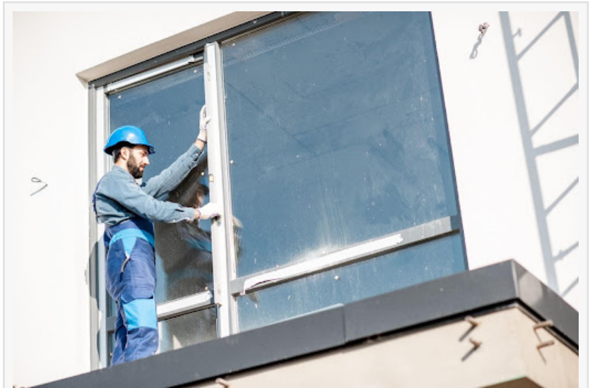
A technician performing an emergency glass repair service professionally mounting a new window to replace damaged glass in a commercial building.
