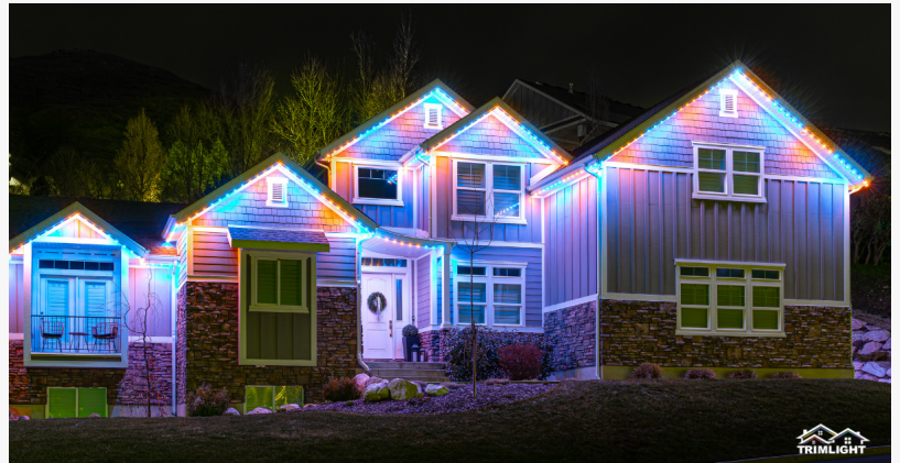
Permanent LED Lights
