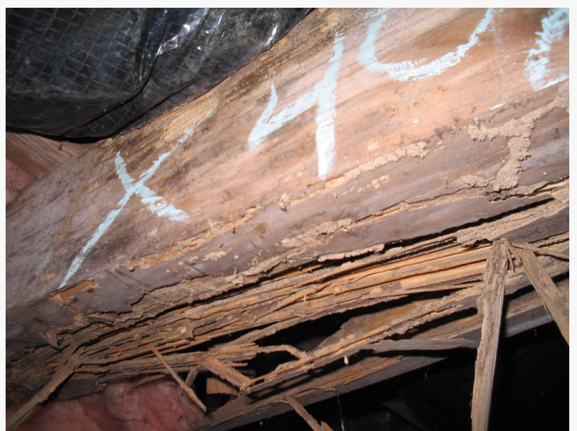
Termite Damage in Virginia Beach
