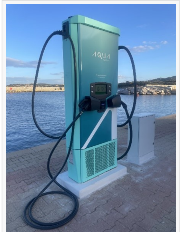
Aqua superPower installation
