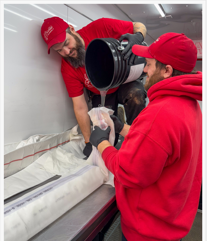
A J. Blanton Plumbing technician performing a trenchless sewer repair, showcasing the company's energy-efficient solutions and expertise as a Lincoln Park emergency plumber offering hydro jetting services.
