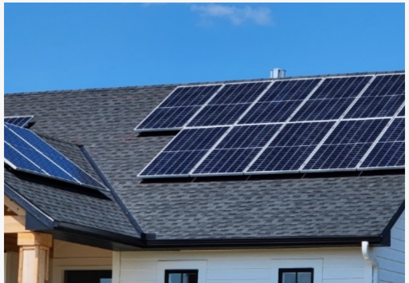
Wolf River Electric Solar Panels in Place
