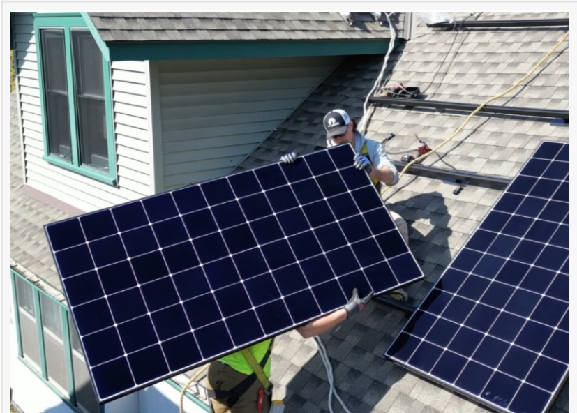
Wolf River Electric Solar Installers
