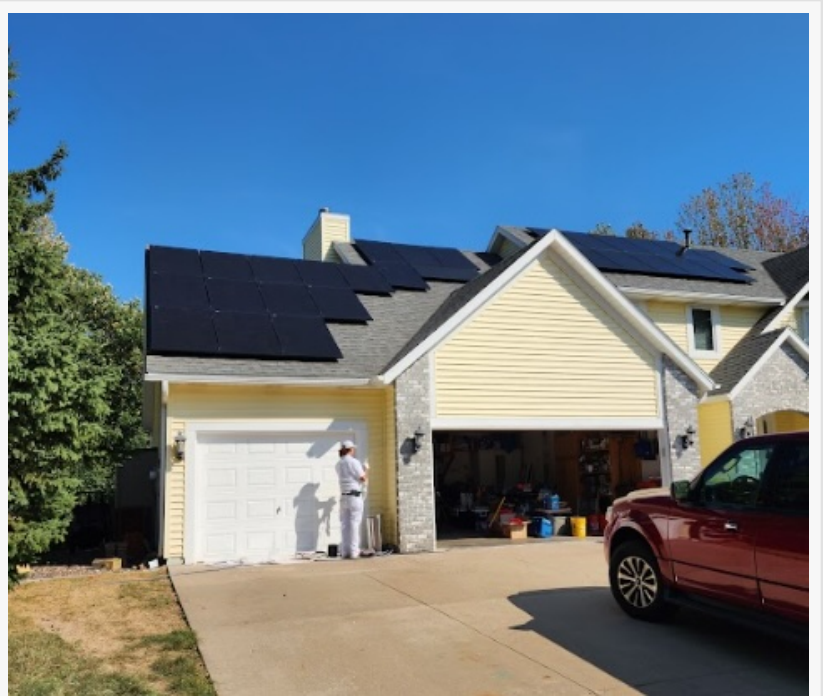
Wolf River Electric Residential Solar Completed
