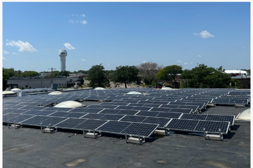
Wolf River Commercial Solar Rooftop
