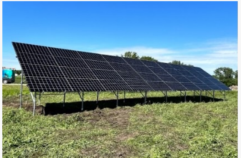
Wolf River Electric Commercial Ground Installation
