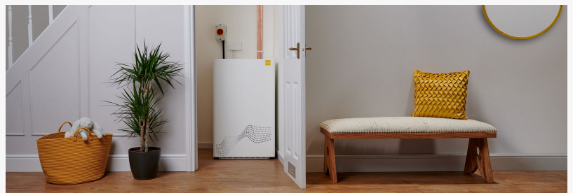
The ZEB under stairs
