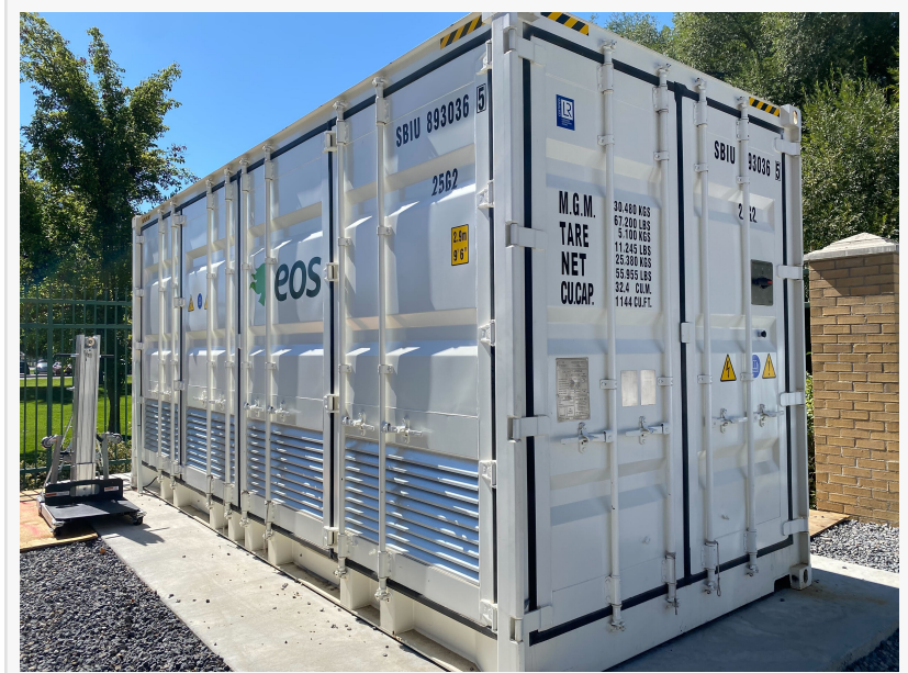
Logan City Light & Power's first energy storage system uses Eos Energy zinc hybrid batteries and a WATTMORE Energy Management System.
