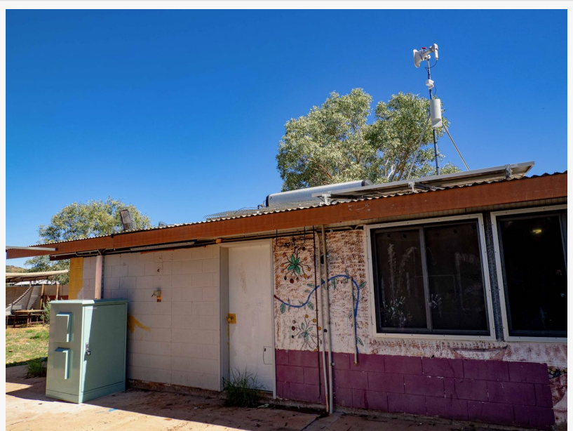
An image of one of the installation sites
