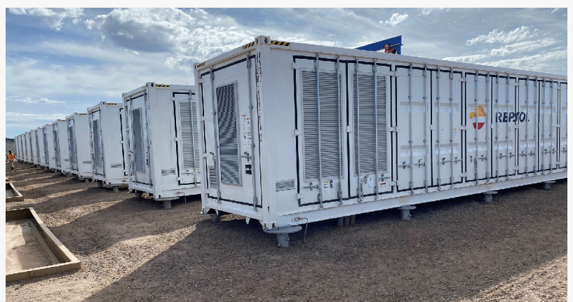
Repsol's 20MW Jicarilla energy storage system in New Mexico
