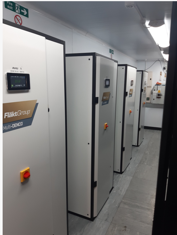
Image of Royal Free Hospital data centre
