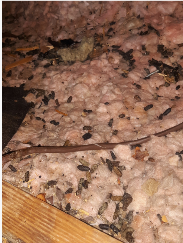
Rodent Entry Point in Vent
