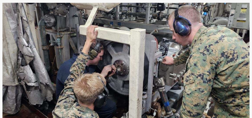
U.S. Navy Machinery Repairman 2nd Class John Jones, left, installs a 3D-printed stainless steel reverse osmosis pump sprocket bushing aboard USS Somerset (LPD 25) with the help of U.S. Marine Corps Lance Cpl. Trevor Connelly and Staff Sgt. Jordan Blake.
