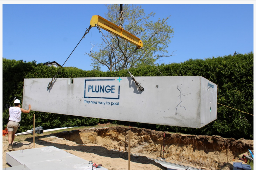
Installation of a Plunge Plus pool from newly formed Easton Select Group, which is focused on national expansion in pool services and backyard leisure.
