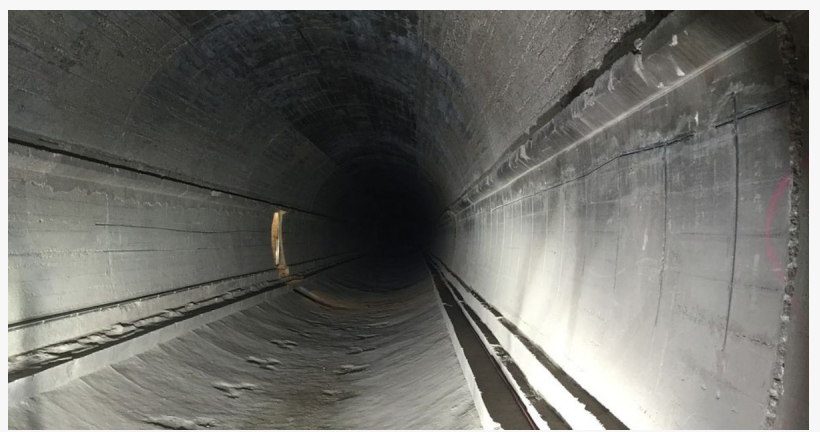
Confined Space Hazards
