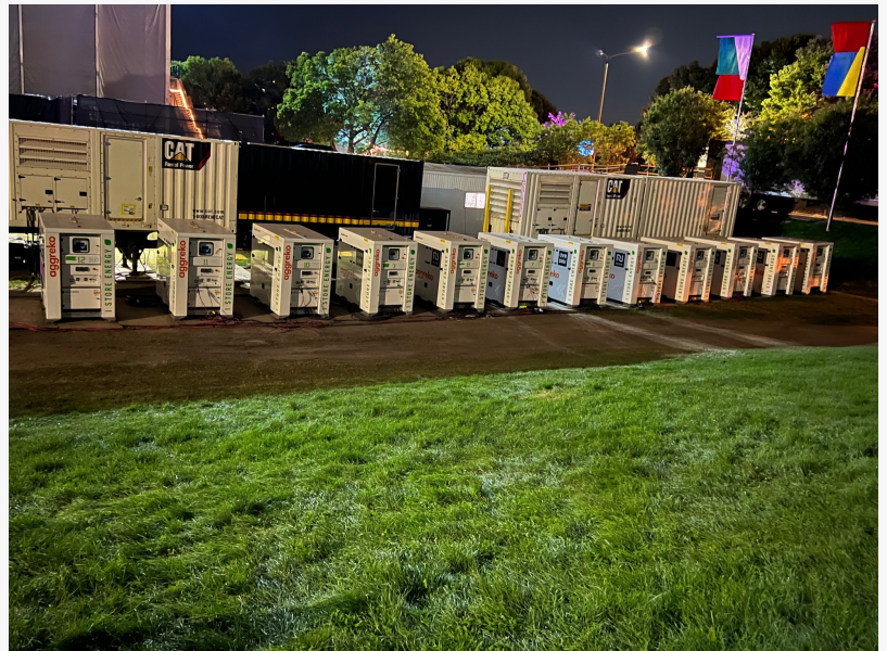
POWRBANKs, charged by a temporary solar array, helped provide clean energy to Lollapalooza's main stage
