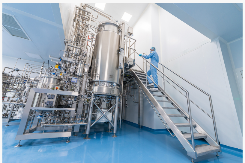
Full view of the 2200 L fermenter in a GMP manufacturing area to produce plasmidDNA biopharmaceuticals
