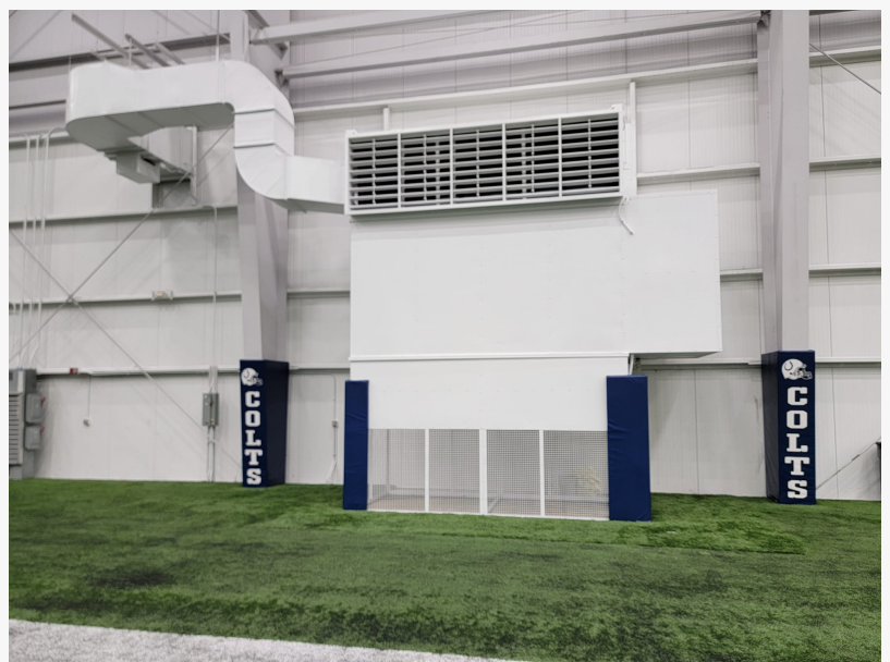
JMI Mechanical Services, inc. HVAC Services for The Indianapolis Colts
