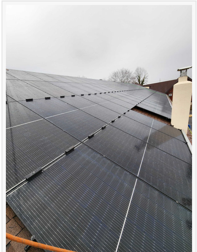
New solar panels on roof of Wakefield Country Day School
