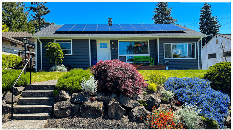
Sunergy Systems Residential Installation
