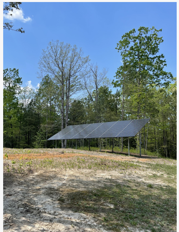
Ground solar array in Toano, Virginia.
