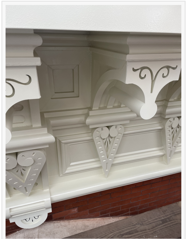
Careful attention to detail and craft ensured a final result worthy of the building's original character and design.
