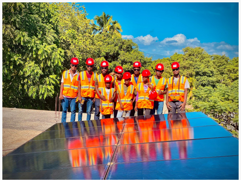
Brighten Haiti Apprentices finish solar installation, providing electricity for the 1st time ever
