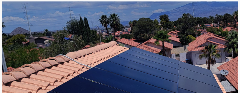
VIG Solar Residential Installation
