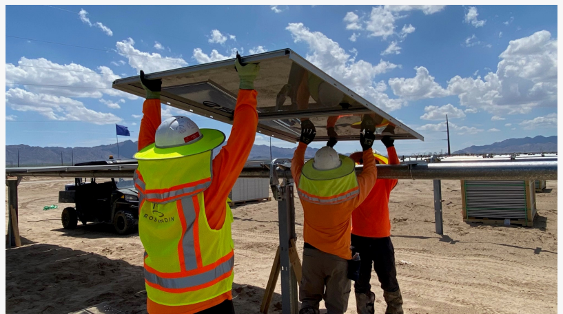
Rosendin installs solar panels at one of the largest renewable energy facilities in California
