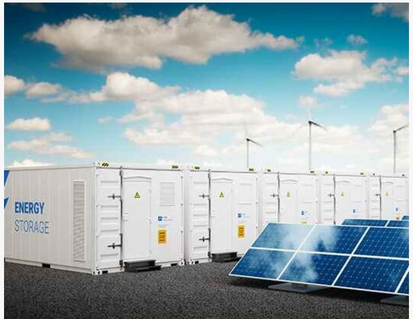
energy storage systems market
