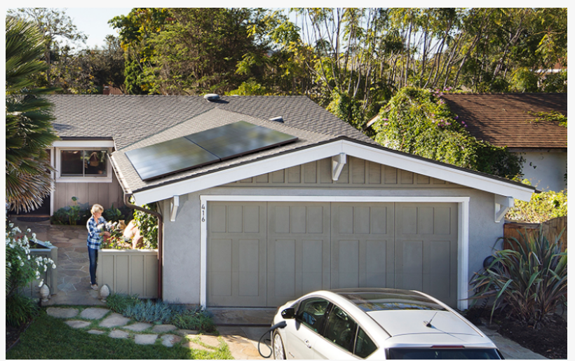
Mirasol Residential Solar Installation
