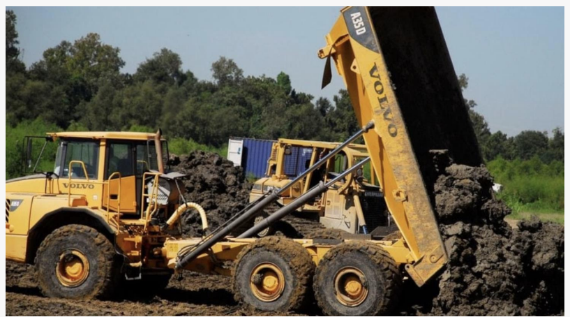
First Lift Levee and Drainage Canal Relocation Project will build levees and drainage canals in Plaquemines Parish
